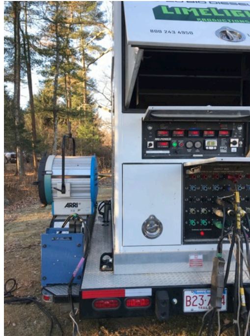
Figure 8: 12kW ghost load on generator to balance load.
