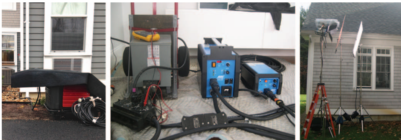
Figure 8 – Covered for rain, a modified Honda EU6500 powers a 4 kW ARRI M40 ARRIMAX fixture through a 60 A transformer/distro.
