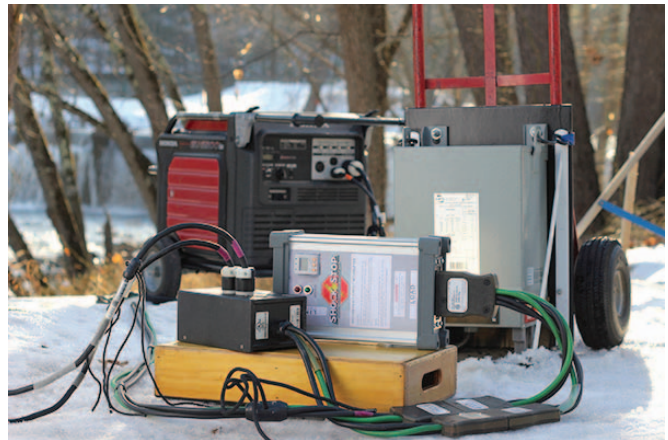
Figure 6 – Shock Stop offers ground fault protection downstream of 60 A transformer/distro
